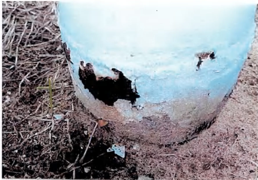
Photograph 1 - Example of piping with Poor atmospheric condition
