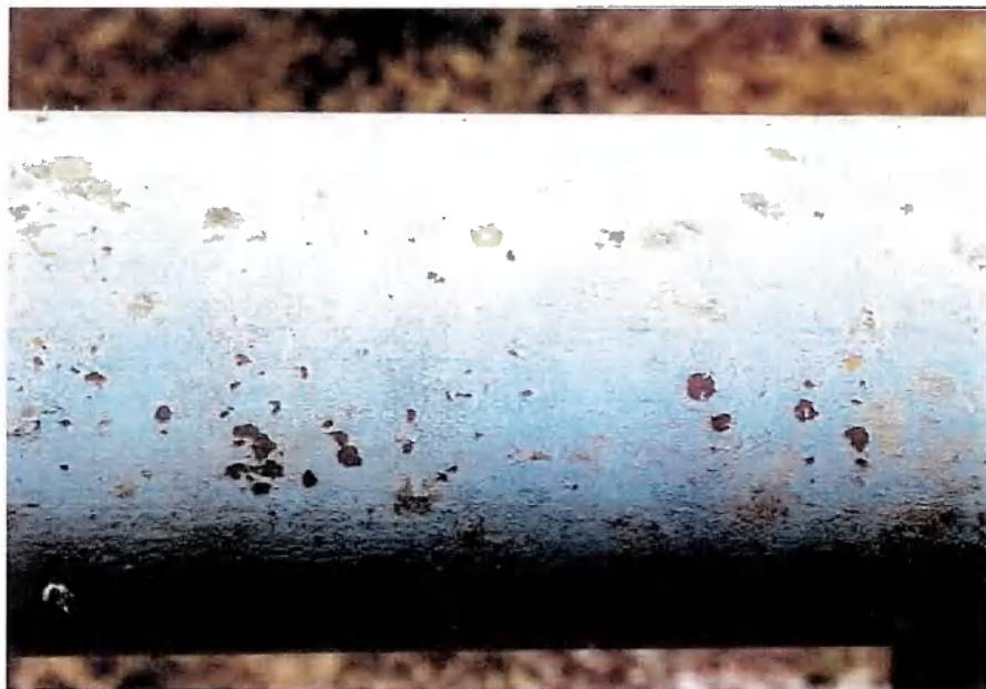
Photograph 2 - Example of piping within limits of Fair atmospheric condition
